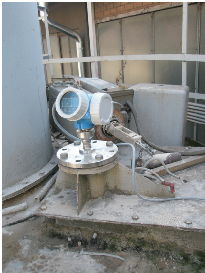
FIGURE 2. A radar level instrument installed on top of a silo.
