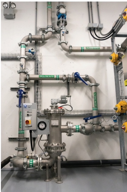
FIGURE 3. This smart pumping application in UV disinfection uses smart instruments to monitor flow control and pump speed to ensure water is passing through the system at precise rates to guarantee quality.
