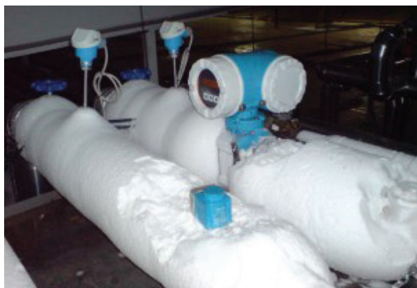
Figure 1: Process cooling and refrigeration systems consume large amounts of energy. Installing flowmeters and other instrumentation helps analyze problems and find leaks
