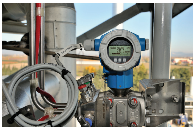
Figure 1: Differential pressure is the most widely used level measurement method in the chemical and petrochemical industries.
