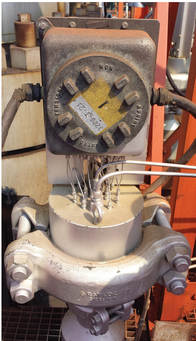
Figure 5: The enclosure at the end of the Flexible Multiplane array thermowell contains transmitters that send sensor data to the control system, or a terminal block assembly that sends sensor data via thermocouple cables to the control system.
