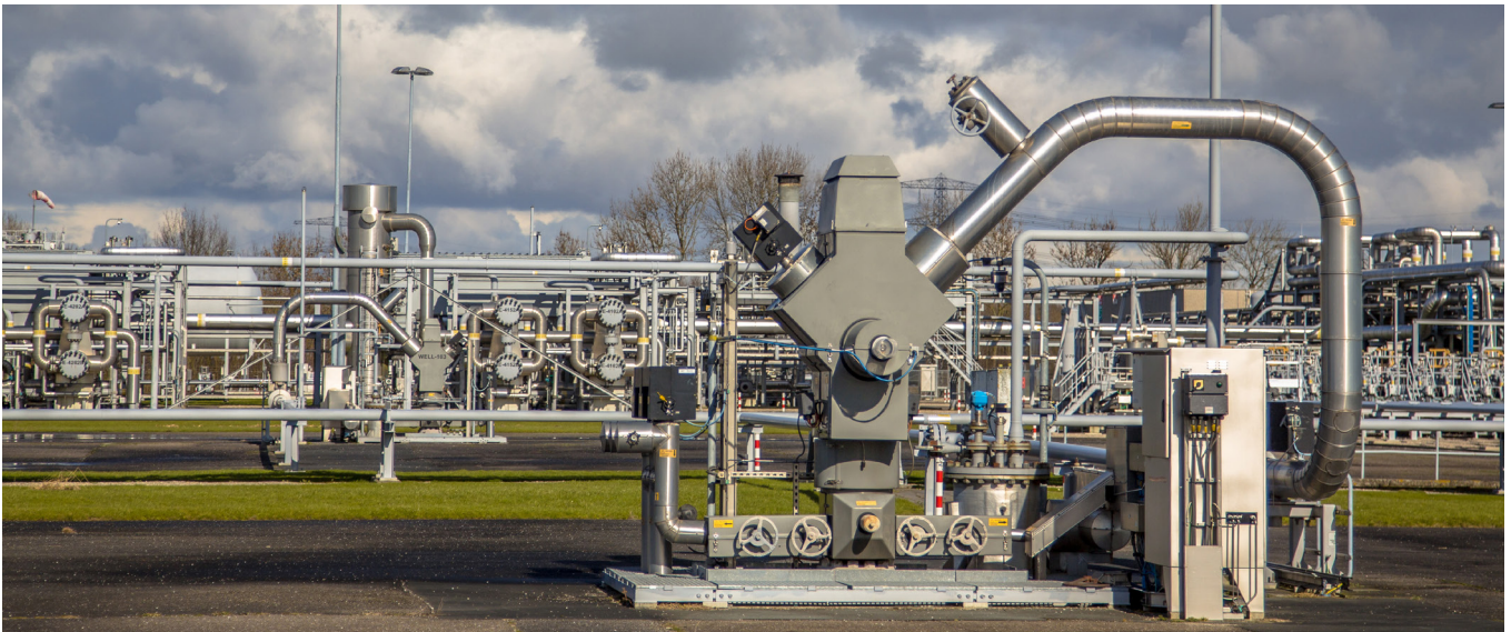
Figure 1: Natural gas well with piping.
