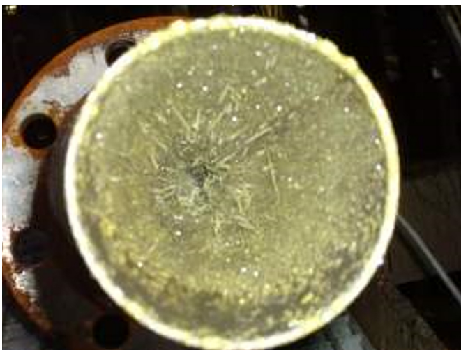
Figure 3: Buildup on free space radar antenna, which does influence the safety function.
