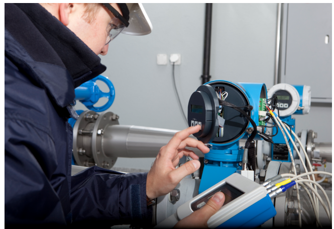
Figure 1: An individual technician can evaluate instruments one by one, but this manual approach can't keep up with a large population of field devices.
