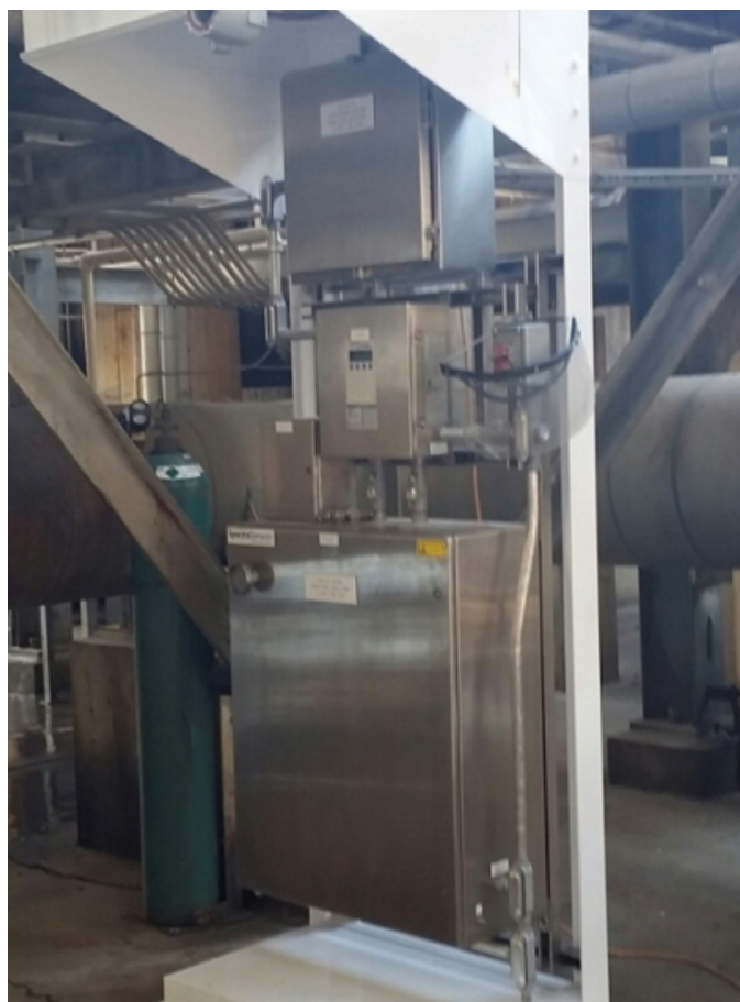
Figure 4: TDLAS analyzers are compact and can usually be field mounted, without the need for elaborate shelters.
