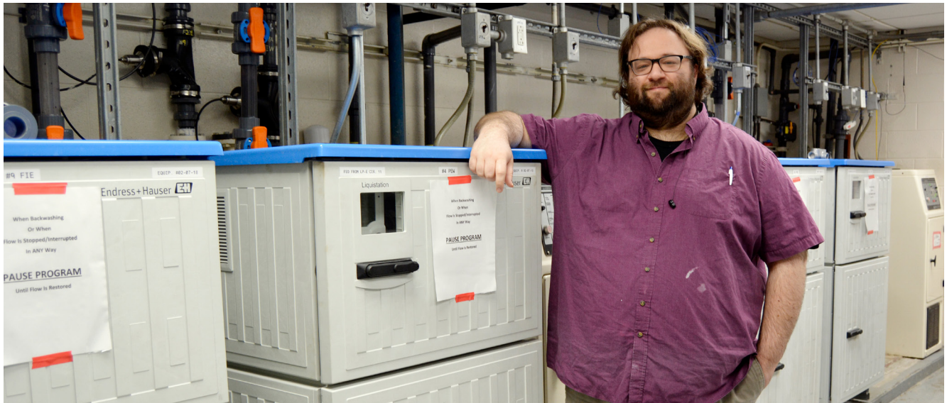
Andrew Hayman (Lab Director for the City of Warren Wastewater Recovery Facility) located in the sampler room. Process from across the plant is diverted here for ease of testing and sample analysis.
