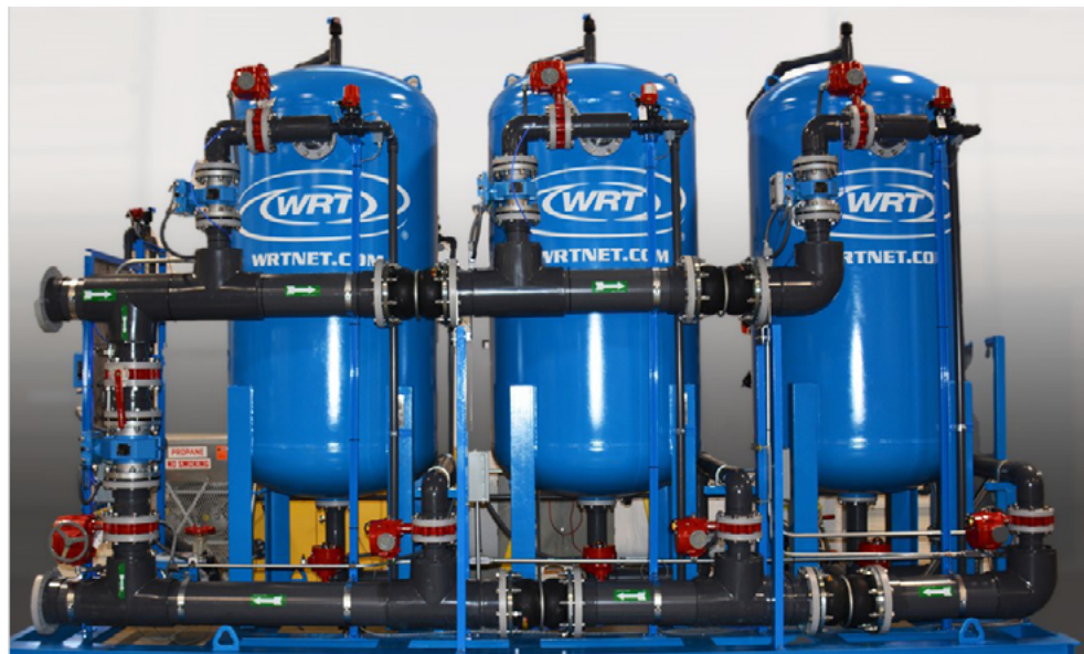
WRT uses Endress+Hauser's Viomax CAS51D digital nitrate sensor and a Liquiline CM444 four-channel transmitter.
