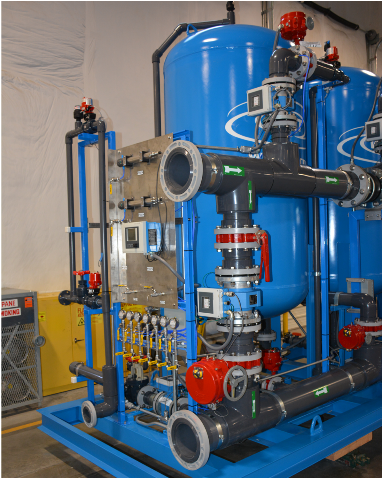
Endress+Hauser's CAS51D and Liquiline transmitter enhanced WRT's nitrate removal system. WRT can now better monitor process steps, fully utilize all the salt they are using and obtain full cycles from media.
