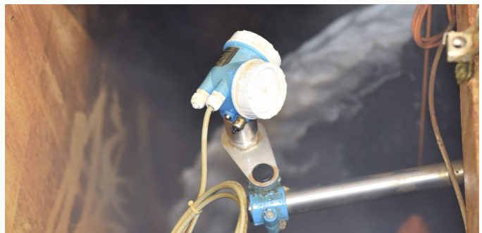
Figure 6: The Micropilot FMR50 radar level sensor by Endress+Hauser can detect foam buildup in wetwells, and this can be used to automatically determine the ideal time and quantities to dose bacteria-stabilizing additives.
