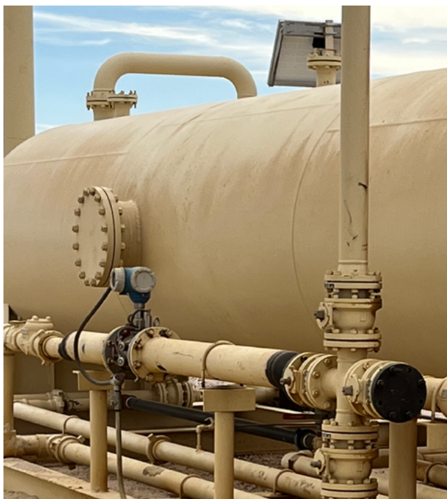
The mixture of oil, water and gas goes through a multi-stage separation process. To allocate fluid components to each well, high quality and reliable instrumentation is needed.
