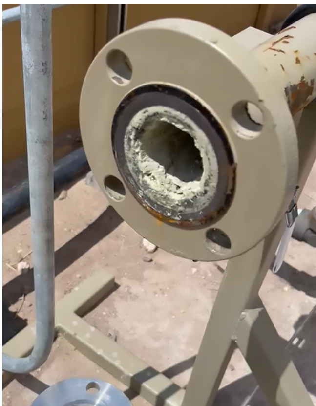
A buildup in gas lines can cause process-interrupting issues. In the case of this company, chemicals used in the well-stimulation process resulted in significant buildup.
